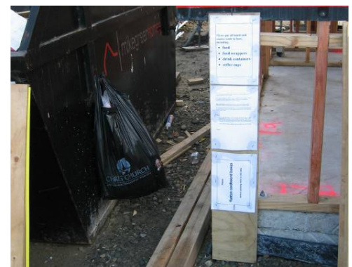
Signs asking sub-contractors to put wet waste in the black bag © Copyright
