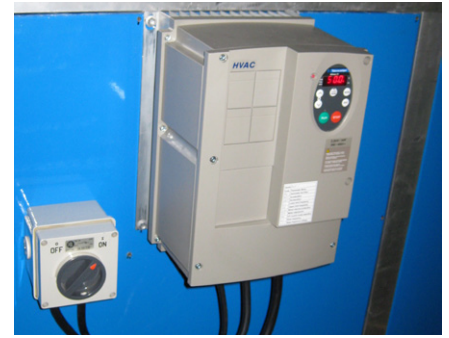
Variable speed drive on one of the AHUs © Copyright
