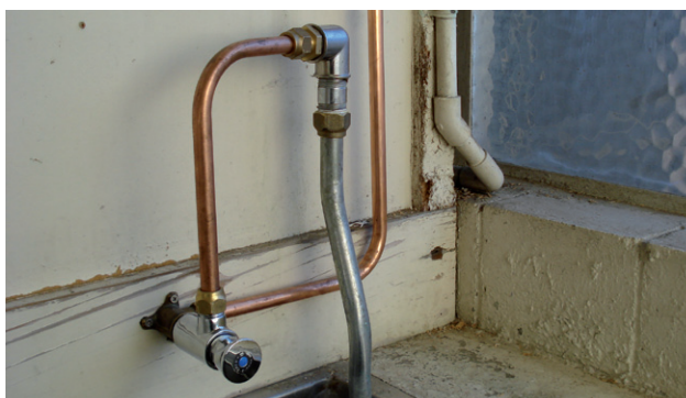
Timed flow valve on the urinal © Copyright
