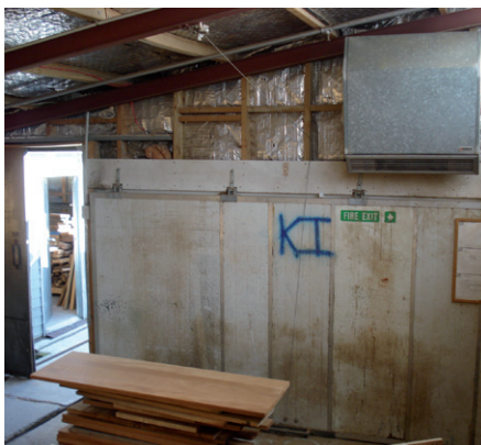
The heater next to the door leading outside © Copyright
