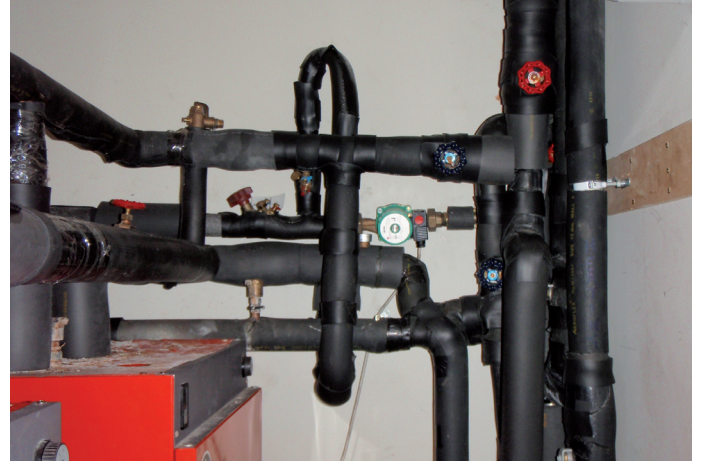
Full hot water pipe insulation lagging was installed to reduce heat loss © Copyright
