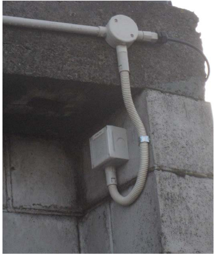
Daylight sensors on the yard lighting © Copyright
